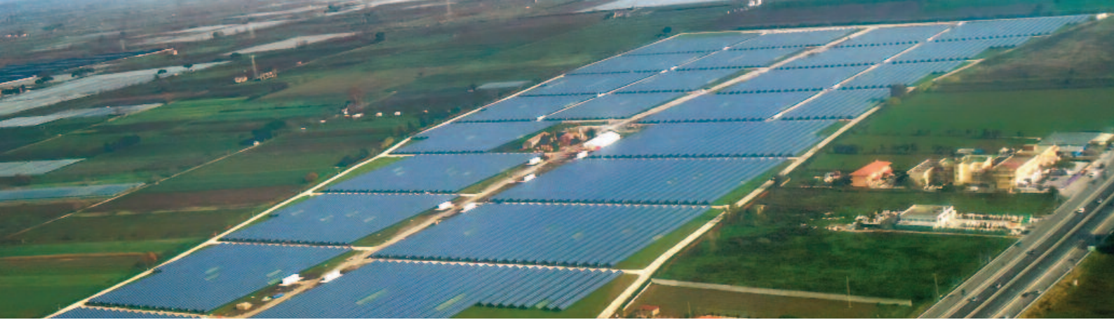
Solar energy park in Campania, Italy.
